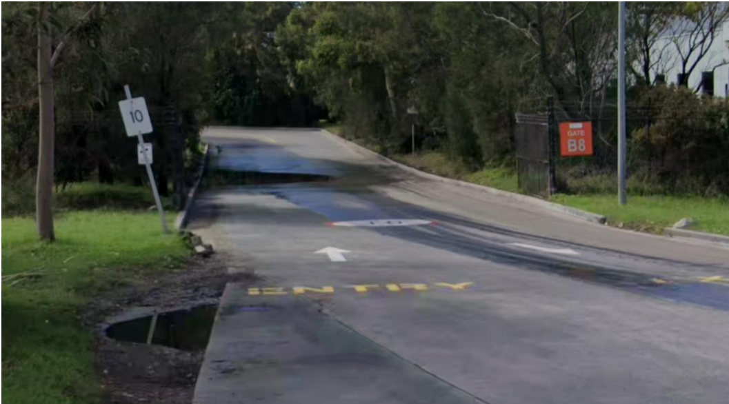
Figure 14: Ponding in Terminal entrance driveway
